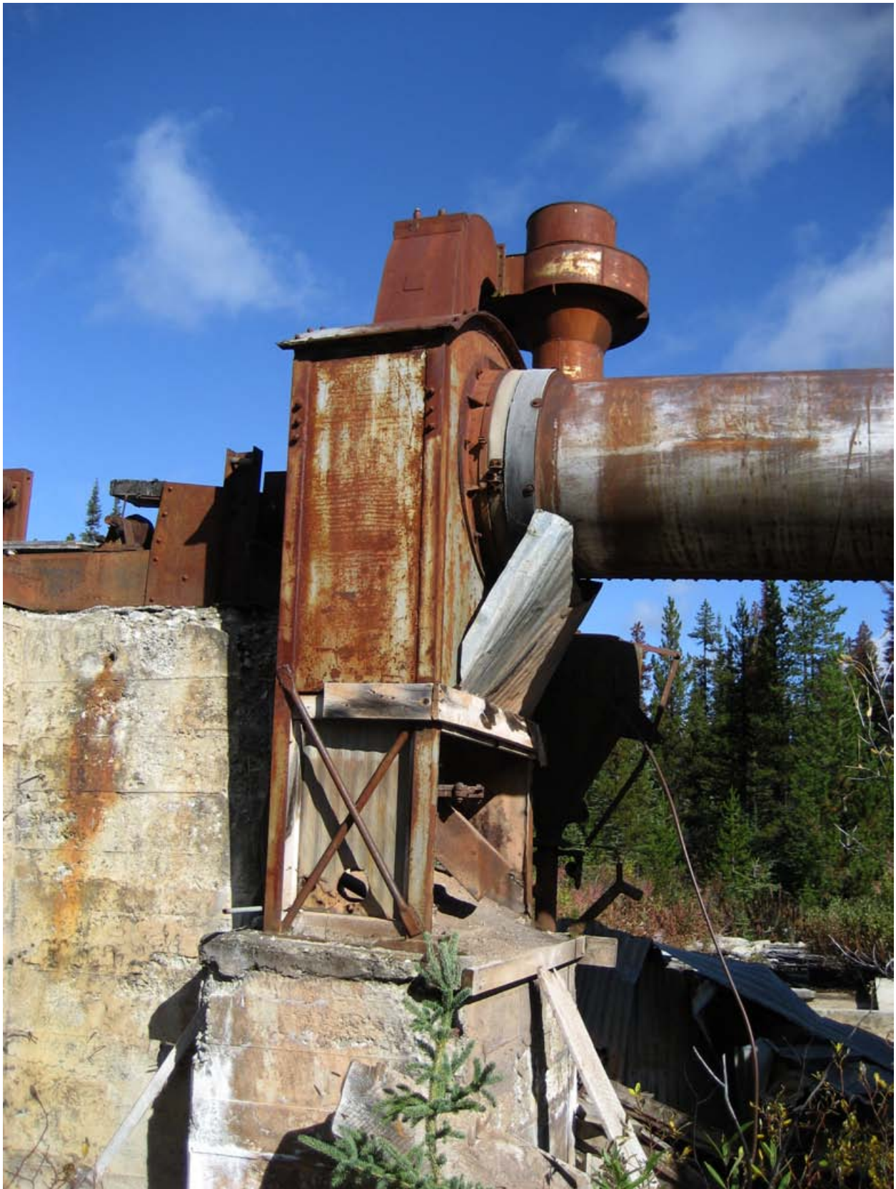
The abandoned Bralorne-Takla Mine, which dates to World War II, still has rusted equipment that was used in mercury mining operations.
